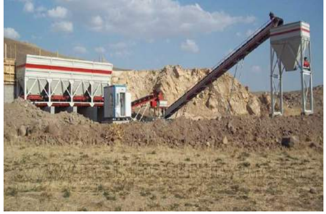
MECHANICAL STABILIZATION PLANT
